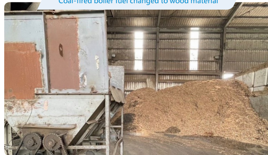
Coal-fired boiler fuel changed to wood material
